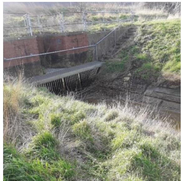
West Tilbury Main at its outfall to the River Thames. South-west view showing the upstream face of Bowater Sluice. Date: October 2019
